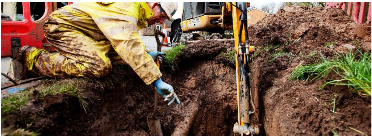
Minimising the amount of water lost through leakage (Photo: Severn Trent)
